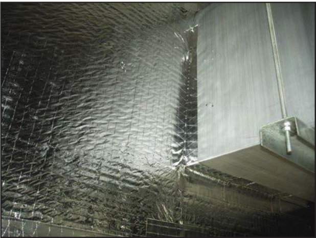
Privacy Board sealed at duct penetration
